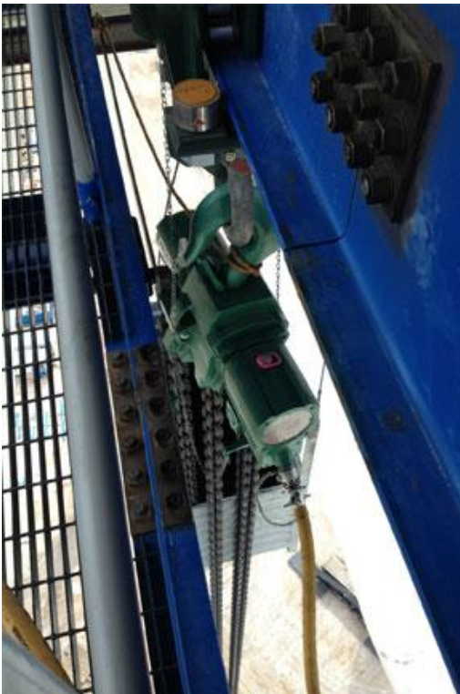
One of three J D Neuhaus air operated hoists mounted at the temporary chain fall platform during construction of the Las Vegas High Roller observation wheel.
