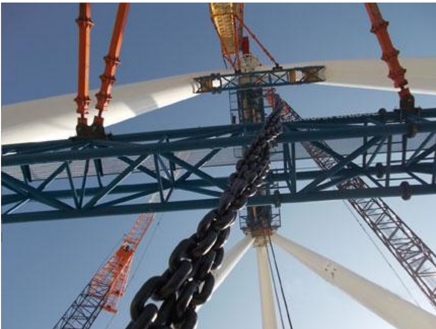
Multiple lines of a J D Neuhaus Air Hoist Chain hang suspended 280ft beneath the chain fall platform down to ground level.
