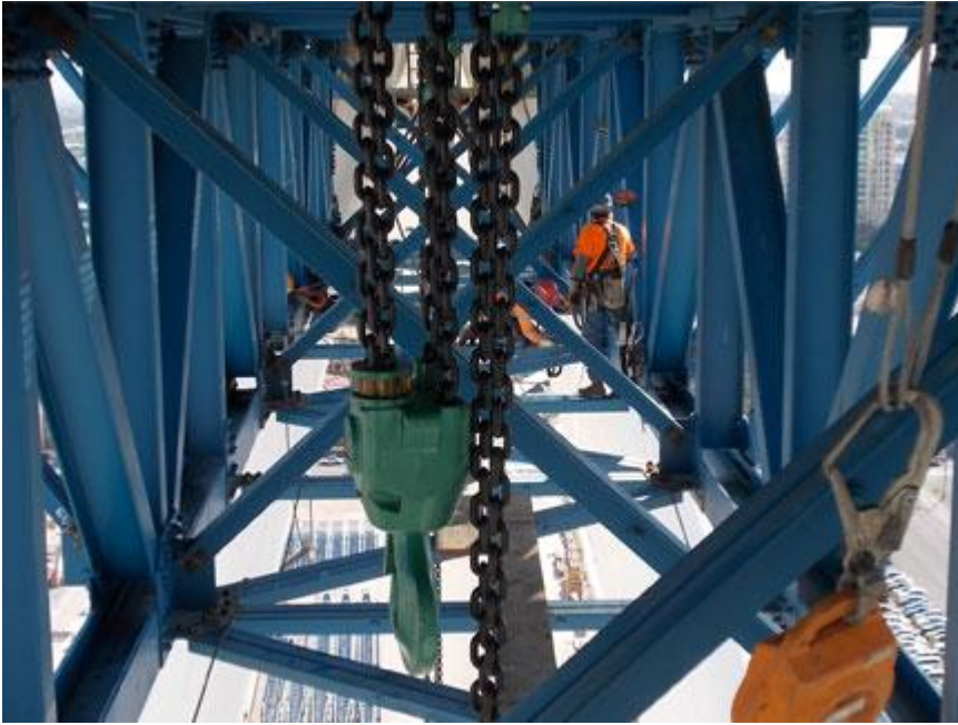
Ironworkers prepare to dismantle the 85 ton hub & spindle transfer truss, first suspending the weight of it from the newly erected chain fall platform above.
