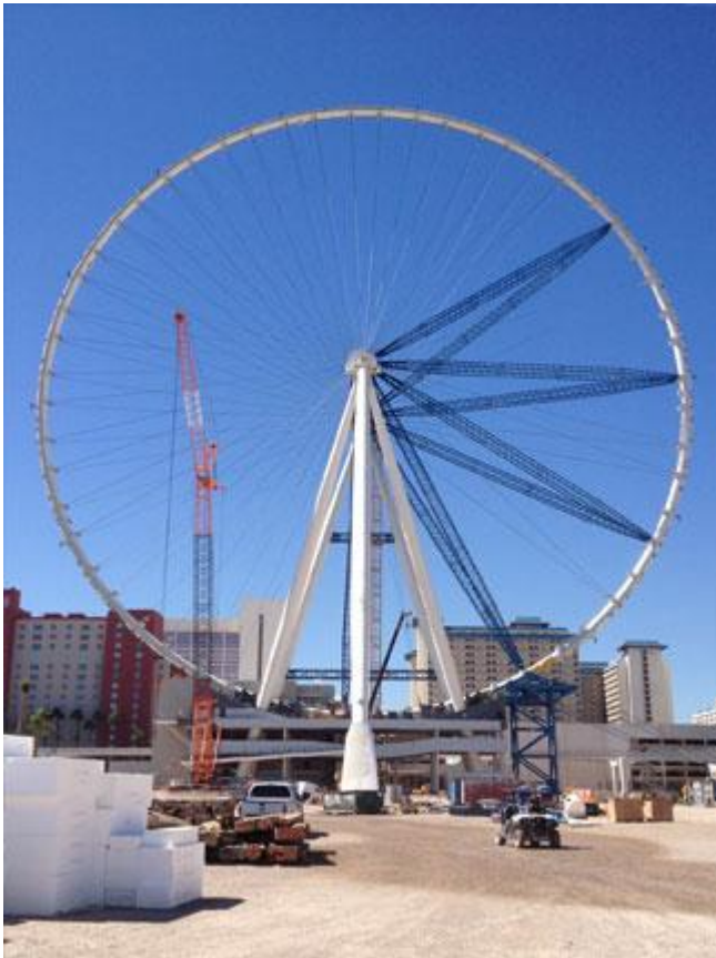
The Las Vegas High Roller observation wheel under construction, showing the outer rim completed with final radial spokes to be added before removal of the temporary radial struts.
